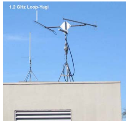
Figure 23 – 1.2 GHz Loop-Yagi receiving antenna on roof of OPD
