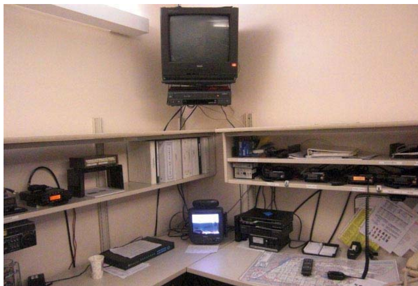
Figure 13 – Inside the COAR RACES Radio Room
