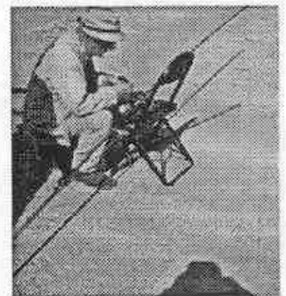
Repair Time for PFA
