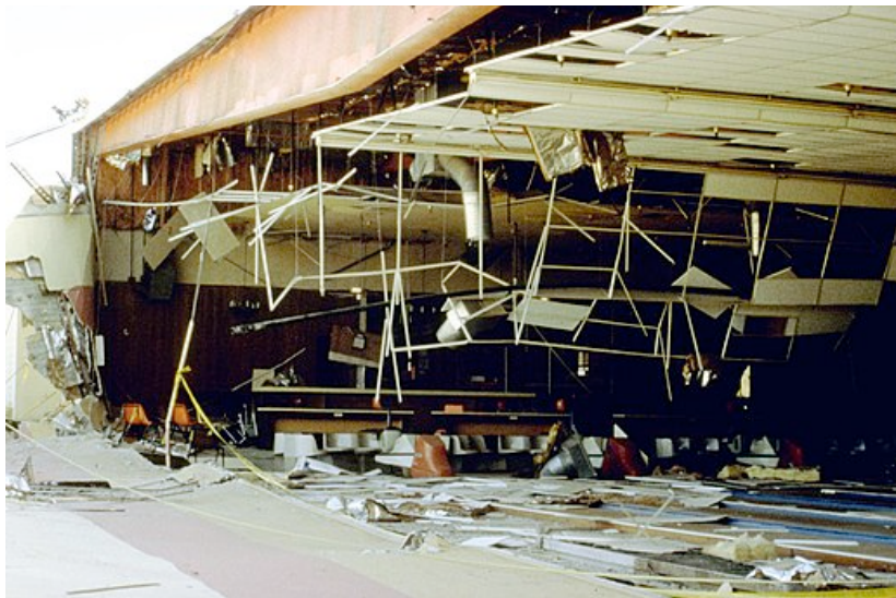
Damage to the Yucca Lanes Bowling Center
