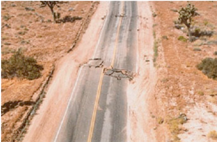
Damage to Highway 274 Image from CalTech Southern California Earthquake Data Center
