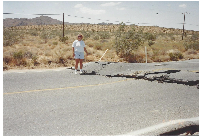
Earthquake rupture along highway 247 (Old Woman Springs Rd)
