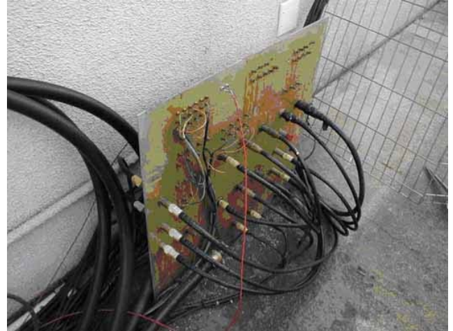
Figure 1 - Grounding Plate for Cables
