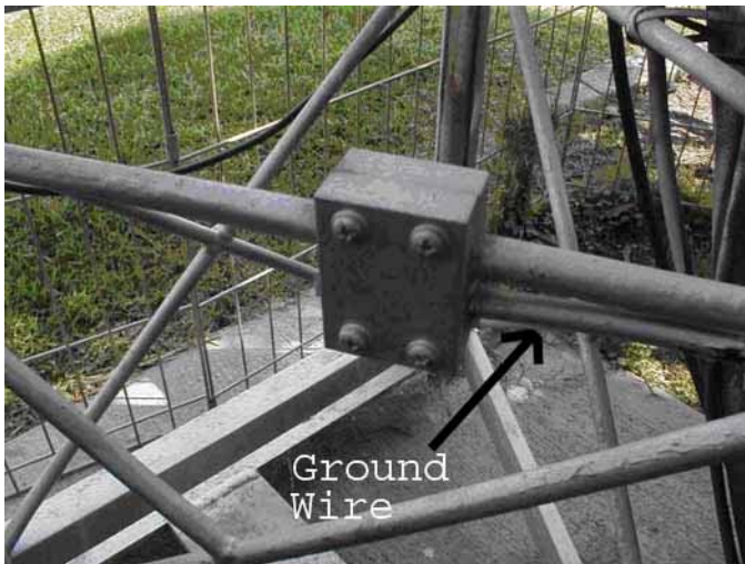
Figure 2 - Shows one way to tie your antenna tower to ground with the use of a tower rung grounding clamp (from ICE Corporation)
