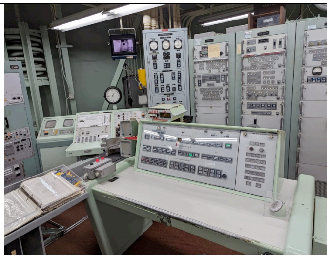
Figure 3 -- Control Room. (Note large spring in background)
